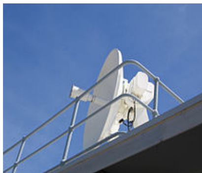
Weather (WF44) radar dish
