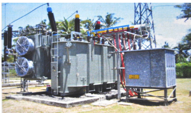
Figure 1.2: The power transformer, Source: Sumatera interconnection system, PLN
