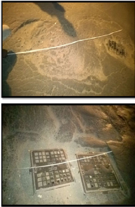
Fig -1: Measurement of Potholes, Drainage Catch Pits Measurement
